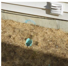
Defective sewer cleanout.
