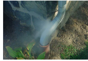
Incorrectly connected downspout.
