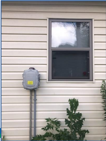
Pictured below: Installed Control Panel
