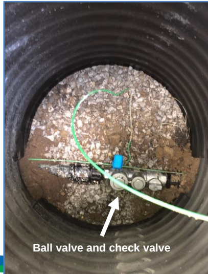
Pictured below: Inside of Service Box/Valve Pit
