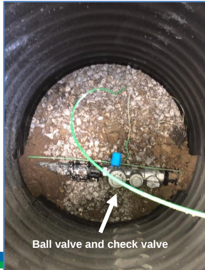
Pictured below: Inside of Service Box/Valve Pit
