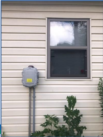
Pictured below: Installed Control Panel
