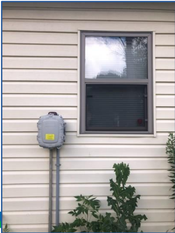
Pictured below: Installed Control Panel
