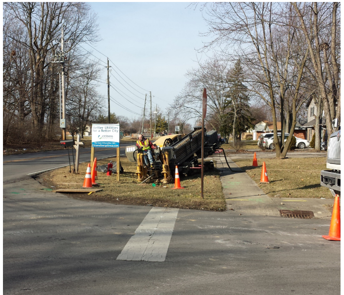
Above: Directional boring machines allow pipe to be installed under streets without disrupting street cutting and excavation.
