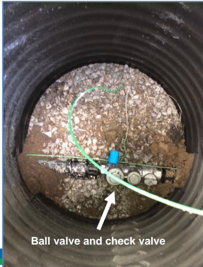
Pictured below: Inside of Service Box/Valve Pit
