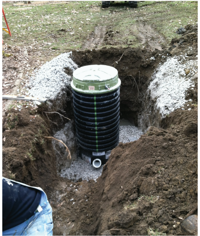
Above: Here is a view of the grinder pump system in the trench. This is prior to piping, refilling the trench with soil and leveling of the site.
