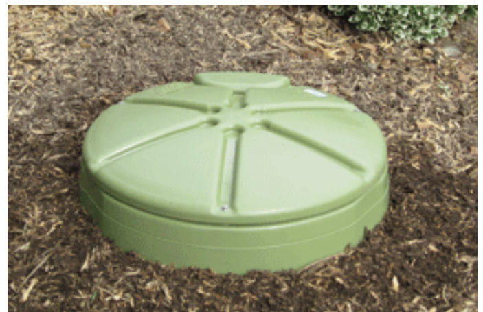
Above: Surface view of the Grinder Pump System (post-installation)
