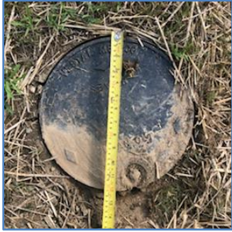
Pictured above: Service Box/Valve Pit Lid
