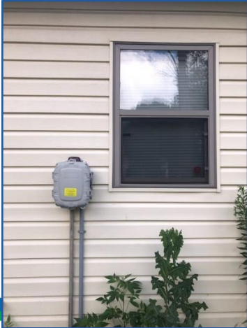
Pictured below: Installed Control Panel
