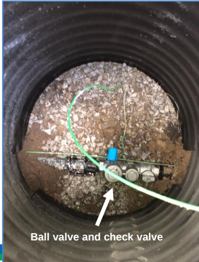
Pictured below: Inside of Service Box/Valve Pit
