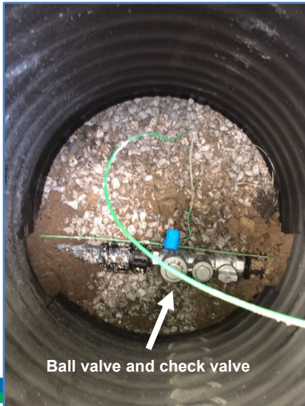
Pictured below: Inside of Service Box/Valve Pit
