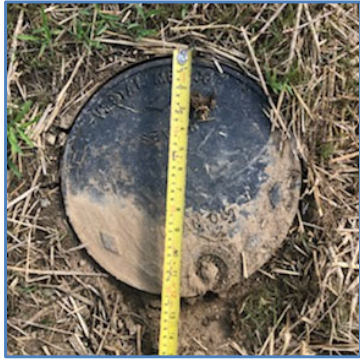
Pictured above: Service Box/Valve Pit Lid
