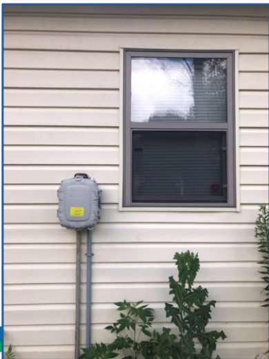
Pictured below: Installed Control Panel
