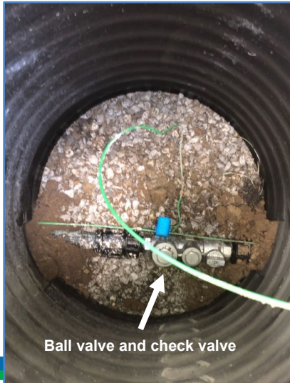
Pictured below: Inside of Service Box/Valve Pit
