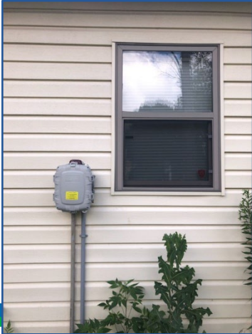
Pictured below: Installed Control Panel
